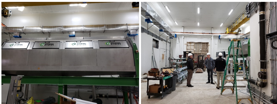
Figure 6. Left: Newly Installed Screw Press for Solids Dewatering. Right: Newly Renovated (Still in Process) Solids Dewatering Room.
