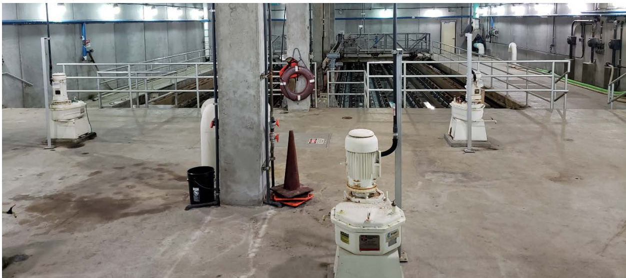
Figure 2. Foreground, flash mix and flocculator mixers. Background, primary clarifiers.
