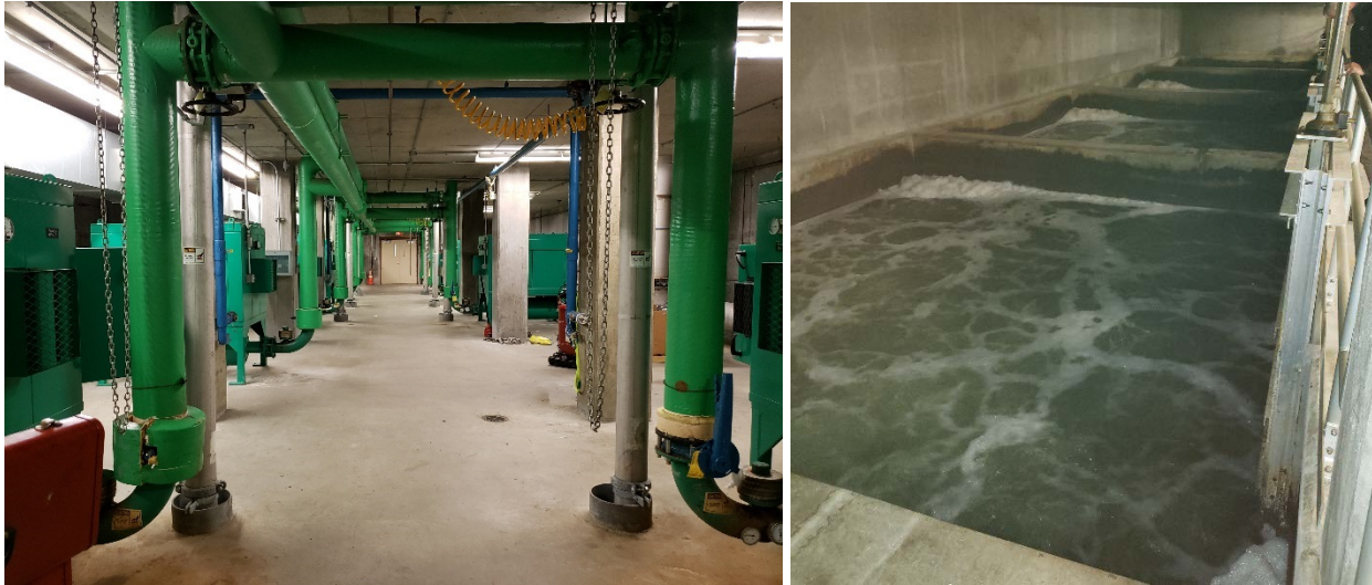
Figure 3. Left: Blower Room. Right: Top of BIOSTYR Cells with Treated Wastewater on Surface.
