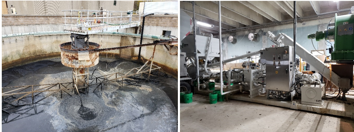
Figure 5. Left: Solids Storage in Decommissioned Clarifier. Right: Temporary Dewatering, Lime Addition, and Reactor.
