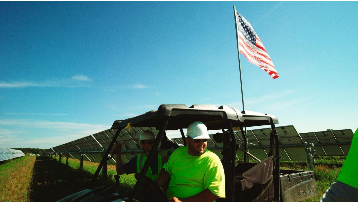
Solar technicians working on site at installation in Chisago County. Credit: The Power of Minnesota (download full resolution photo at http://on.mncerts.org/eawpics )
